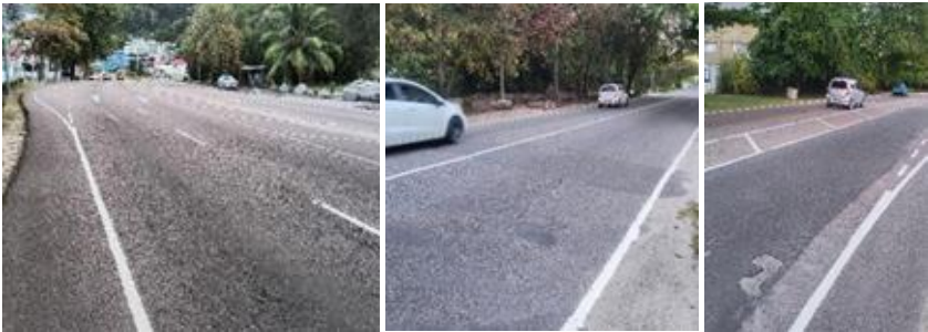
Providence Painting of central median line from Sunshine House to roundabout that had faded away due to heavy traffic flow.
